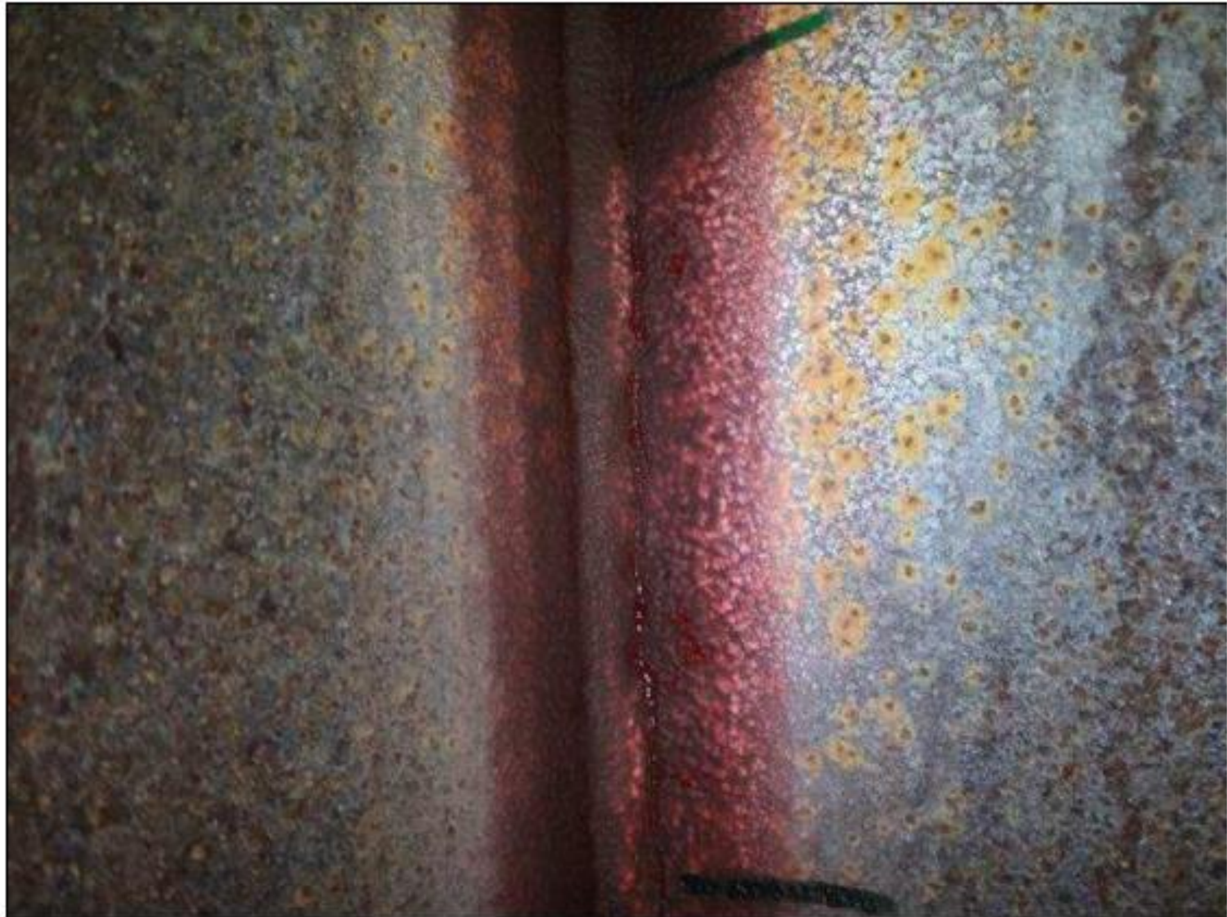
Span 2 Beam 2: upper web to 4th web stiffener from bent 2 exterior face, crack in weld (5in) found after dye-penetrant test performed (photo 1 of 2)
