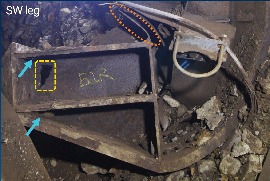
Corrosion product build-up
