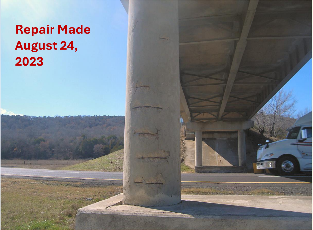
NBI #: 17566 Str #: 5032 0575 XF Facility Carried: I-35 FRONTAGE RD. 2023-02-09 Murray I-35 Feature Int.: I-35 UNDER Pier 2
