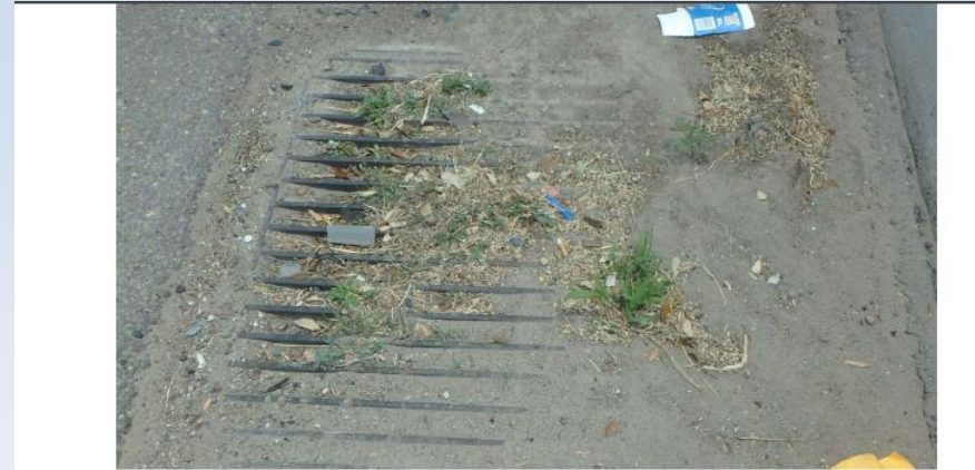
PHOTO 1 Recommended Maintenance Needs Description 21-109-0039-18-282 VIEW 8 - TYPICAL CLOGGED DRAIN INLET AT APPROACHES ALONG SOUTH SHOULDER
