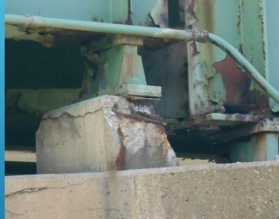
Steel members (girders, crossframes, diagonals etc.) at the supports where expansion joints are located showed surface rust and section loss.
