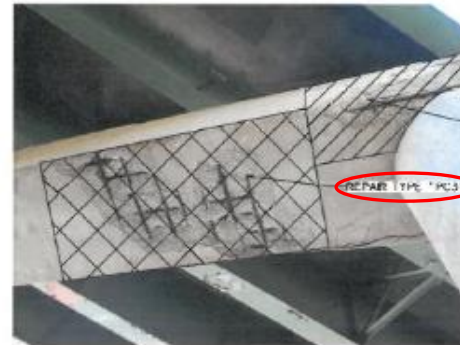
NB PIER 3, BOTTOM OF PIER CAP BETWEEN MIDDLE COLUMN AND WEST COLUMN
