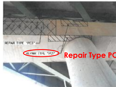
NB PIER 3, BOTTOM OF PIER CAP BETWEEN EAST COLUMN AND MIDDLE COLUMN
