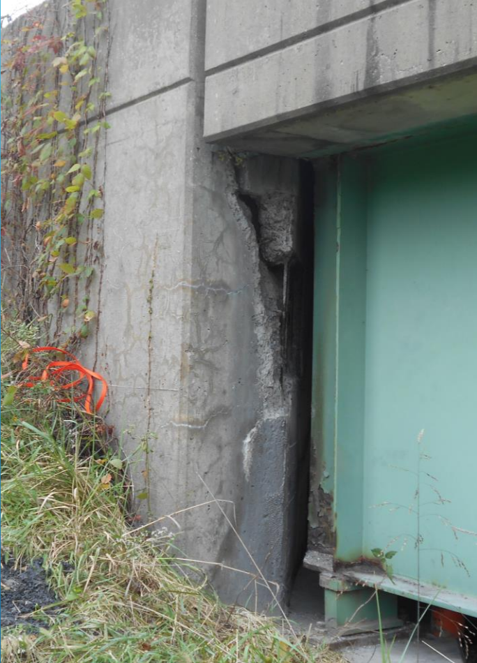
Large spall - A huge chunk of concrete cracked and about to fall off at the corner of Abutment 2, SB structure. Spalls found on all Abutment backwalls in general.
