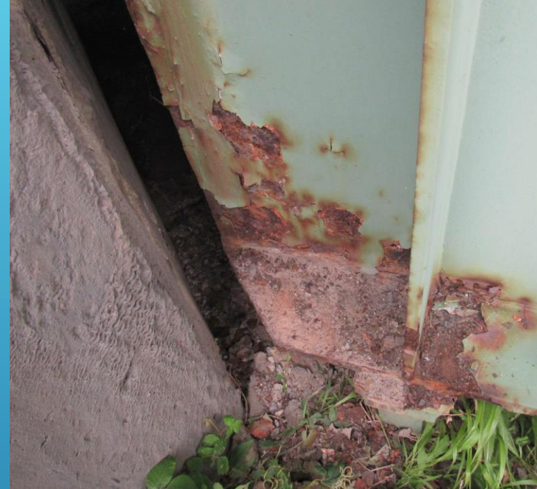
Surface rust and minor section loss at Abutments.
