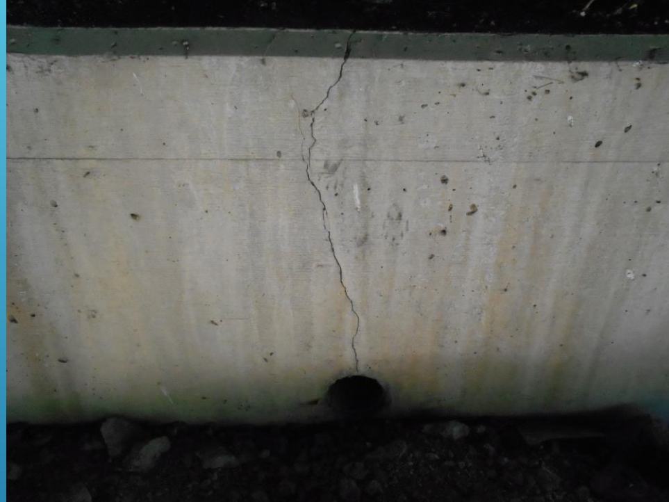
Numerous cracks. Cracks over .03 inches in width were sealed by an epoxy crack sealant.
