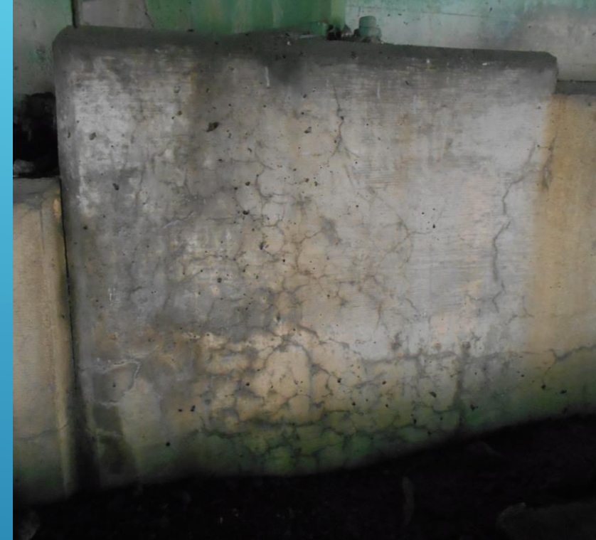
Map cracking. Cracks were sealed off with concrete protective coating
