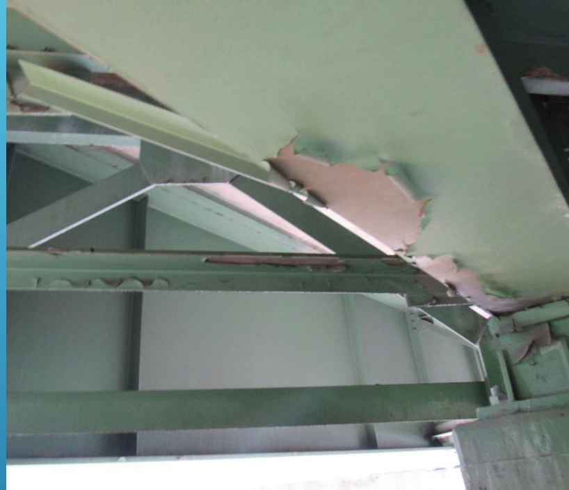
Peeling topcoat on the beam bottom flanges and diagonals. (Pier location)
