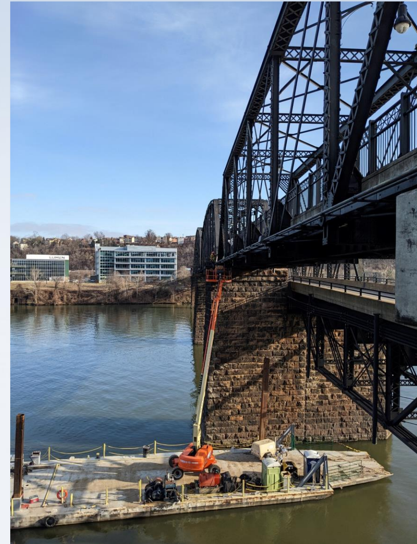
Hot Metal Bridge – Rail to Trail conversion in 2007, first time inspection in 2022!
