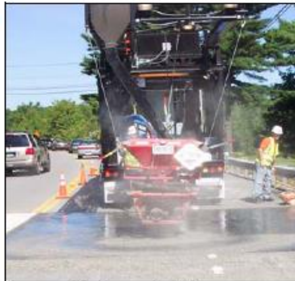
Aggregate is carried from hopper by conveyor and distributed over the epoxy.
